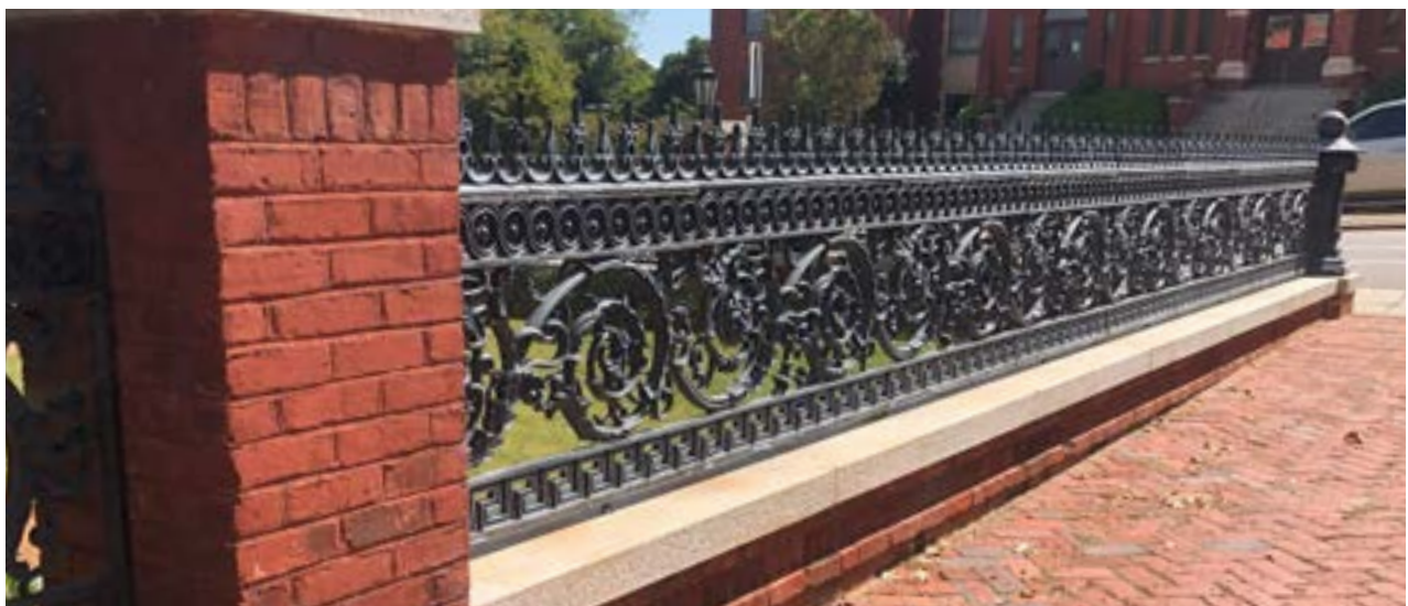
Figure 2.21. This combination fence in the OWE has a masonry base and wrought iron cresting.
