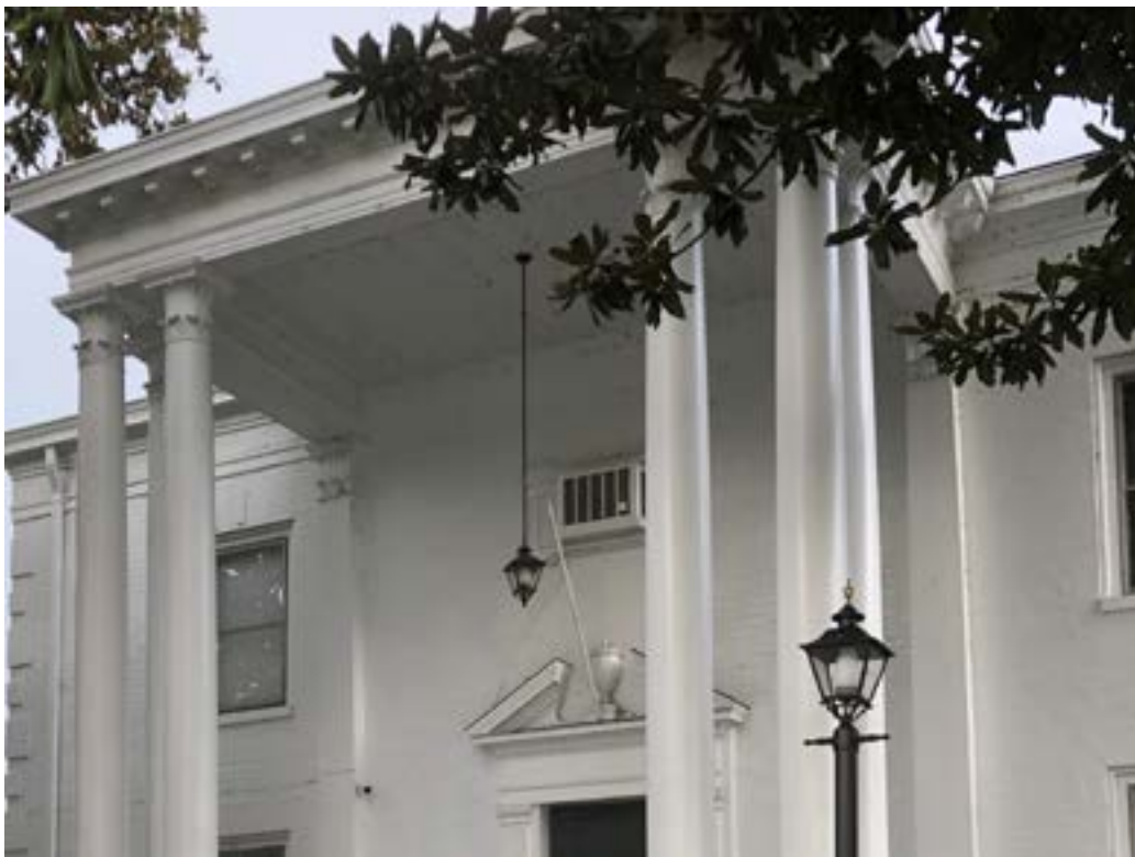
Figure 2.23. Although the placement of a wall air-conditioning unit on the façade is not ideal, the equipment does not obscure any architectural features, has been painted to match the dominant wall color, and is partially obscured by the portico.
