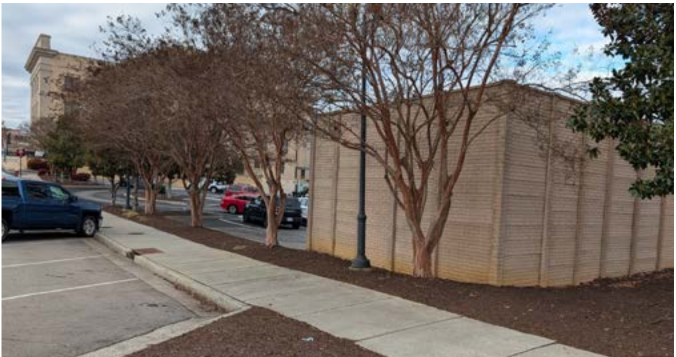
Figure 4.17. Transformers and their concrete pads should be relegated behind buildings and structures, preferably on rear or side elevations of buildings. If that is not possible, transformers and similar utilities equipment should be screened from view from the public right-of-way with an opaque enclosure (such as fencing) or with adequate landscaping.
