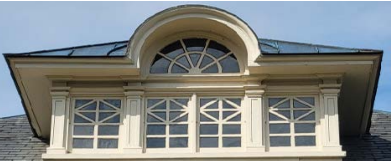
Figure 2.10. Dormers are structural elements, typically with windows, that project above the roof and add living space to the uppermost floor.
