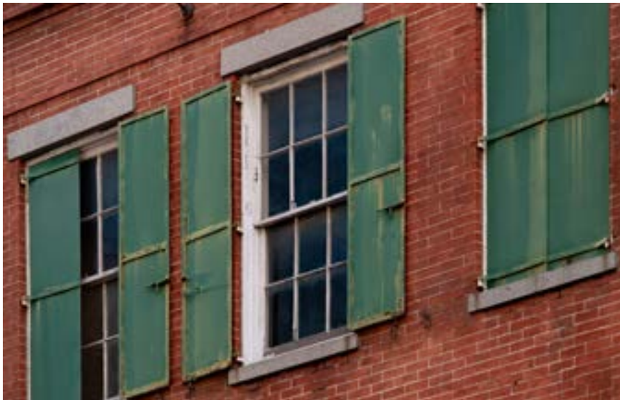
Figure 2.18. Exterior shutters must be operable and fit the window or door opening.
